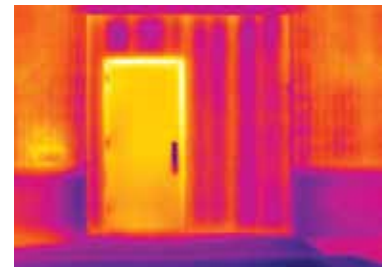
Air leakage: Identify sources of energy loss due to improperly installed or worn seals on windows and doors.
