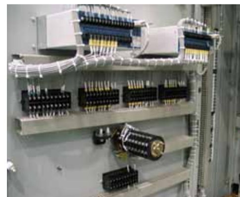
FMS Test Switches used in enclosure
