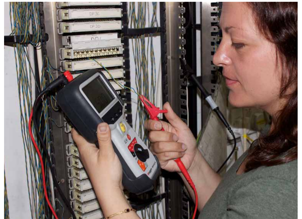
Evaluate circuits in a main telephone distribution frame using a specialised insulation tester. Make sure you specify a 500 V tester to detect moisture induced insulation breakdowns in dry conditions.
